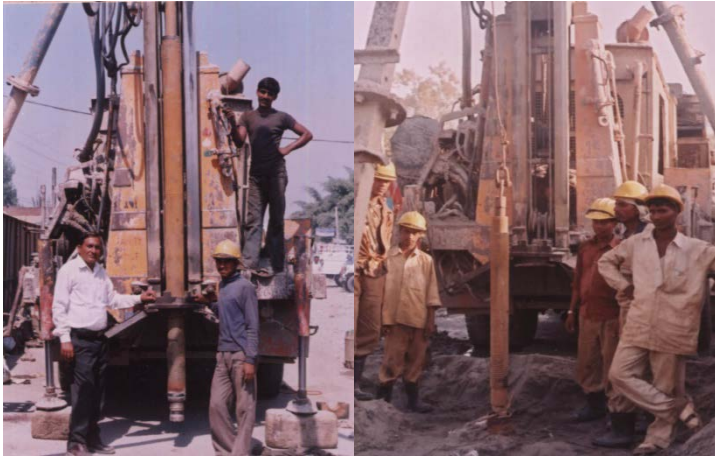
Fig.5: Borehole drilling in progress. Left: Drill bit for odex drilling. Right: Bailer being used to clean borehole prior to conducting SPT
