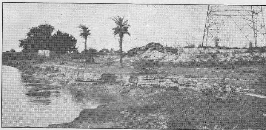
Fig 1 : Foundations Of Existing Transmission Towers Threatened By The Meandering River Yamuna.
